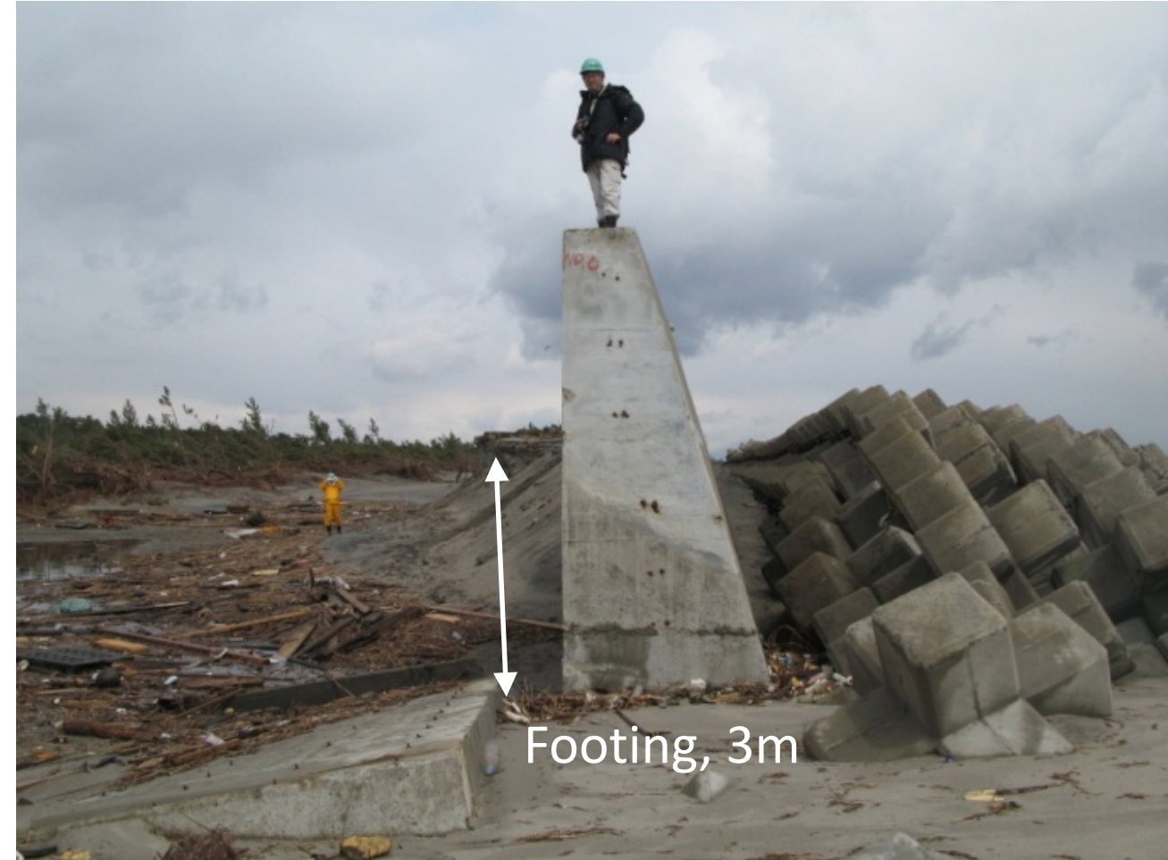
Scouring at Fujitsuka by the 2011 tsunami
